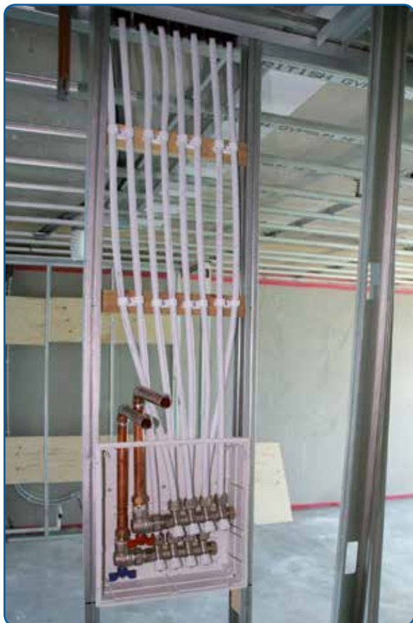
A complete manifold set, the Multiplex is shown here. This has been pressure tested and is ready to be plaster boarded in.
